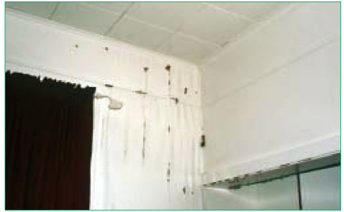
Figure 12. Shelter tubes on interior walls.
