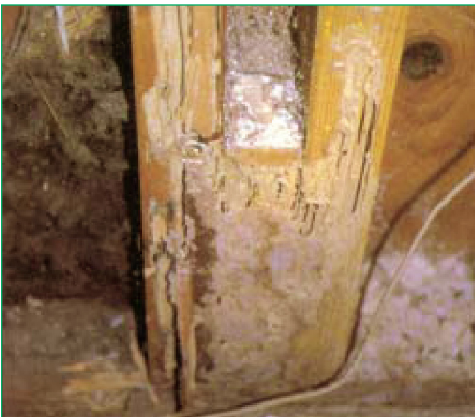
Figure 8. Formosan termite-produced carton nest in a structure.
